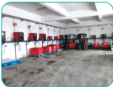
Forklift Charging Room 叉車充電間
