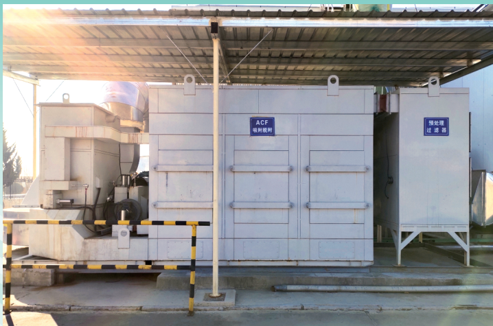
Organic Waste Gas Catalytic Combustion Purification Device
